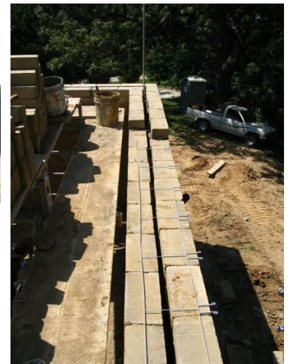
Double wall prior to insulation -Dur-O-Wal lattice tying the two walls together
