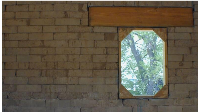
Figure 2 Wood lintel over framed rough opening for window in an unfinished wall
